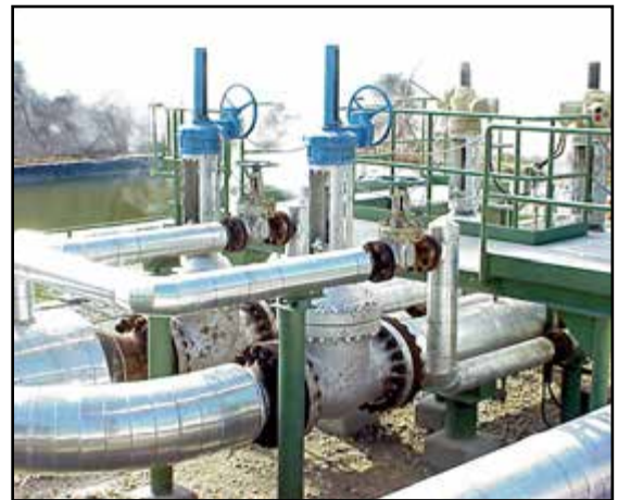
A geothermal power plant valve installation for sour gas service.
