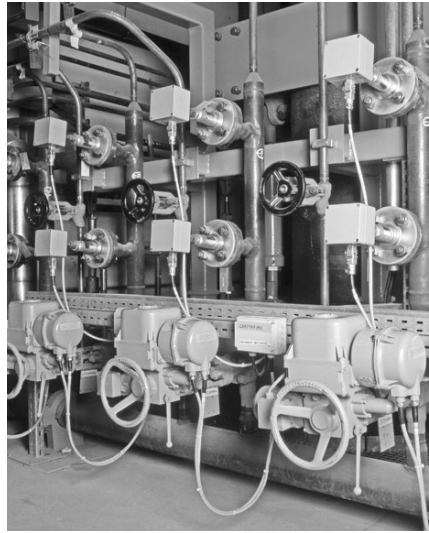
Drain control station using ZK 29 valves with electric actuator
